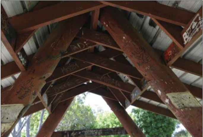
Some of the vandalism damage to the picnic shelter
