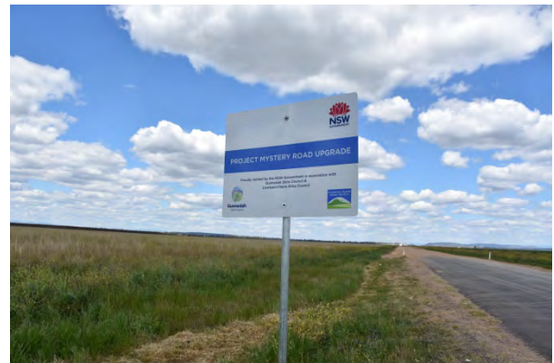
Works completed on the upgrade of Mystery Road near Breeza. Mystery Road is an important link between cotton growers around Carroona and Carroll Cotton in Gunnedah Shire. The upgrade included reconstruction, widening and sealing of 8.1km of Mystery Road.
