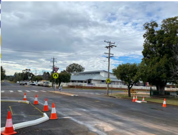
Work commenced making the Bloomfield and Henry Street crossings safer for school children accessing St Xaviers and St Marys College
