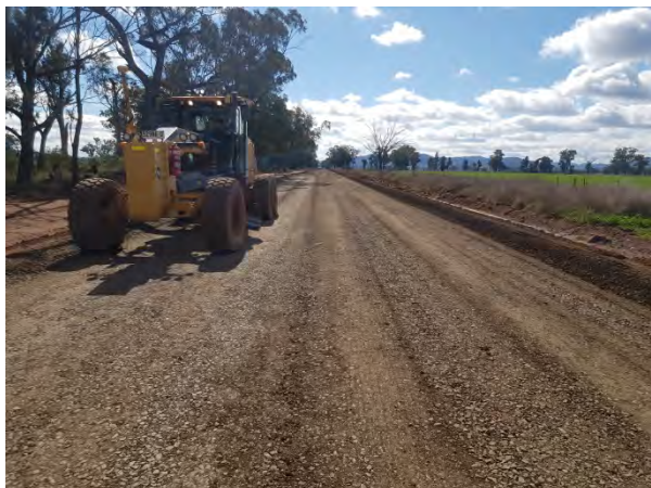
Work commenced on the upgrade of Clifton Road between Carroll and Breeza, with $8.5 million allocated for the upgrade and sealing of 13.5km through the NSW Government Fixing Country Roads Program
