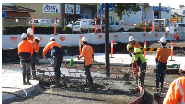
Council staff and contractors commencing work on the Second Rail Overpass Project.
