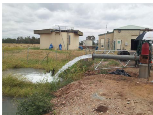
No 8 bore on Orange Grove Road.
