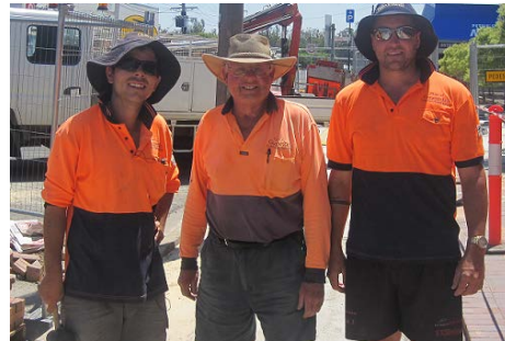
Council's Urban Paving Crew: Kyle Atkinson, Roger Carter and Jacob Mallan working on the footpath paving in Marquis Street.
